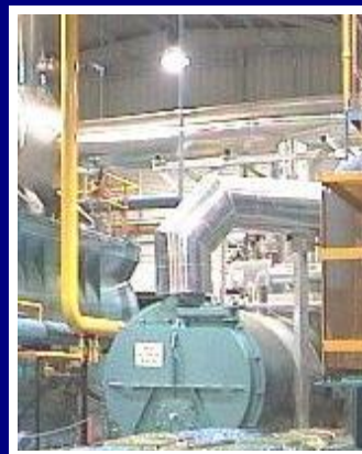
↑ Energy Utilization Heat Exchanger – steam boiler
